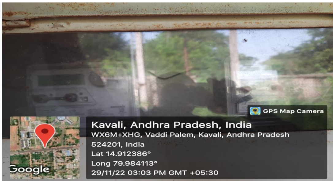
Figure: Grid Connected Solar Plant Net Meter
