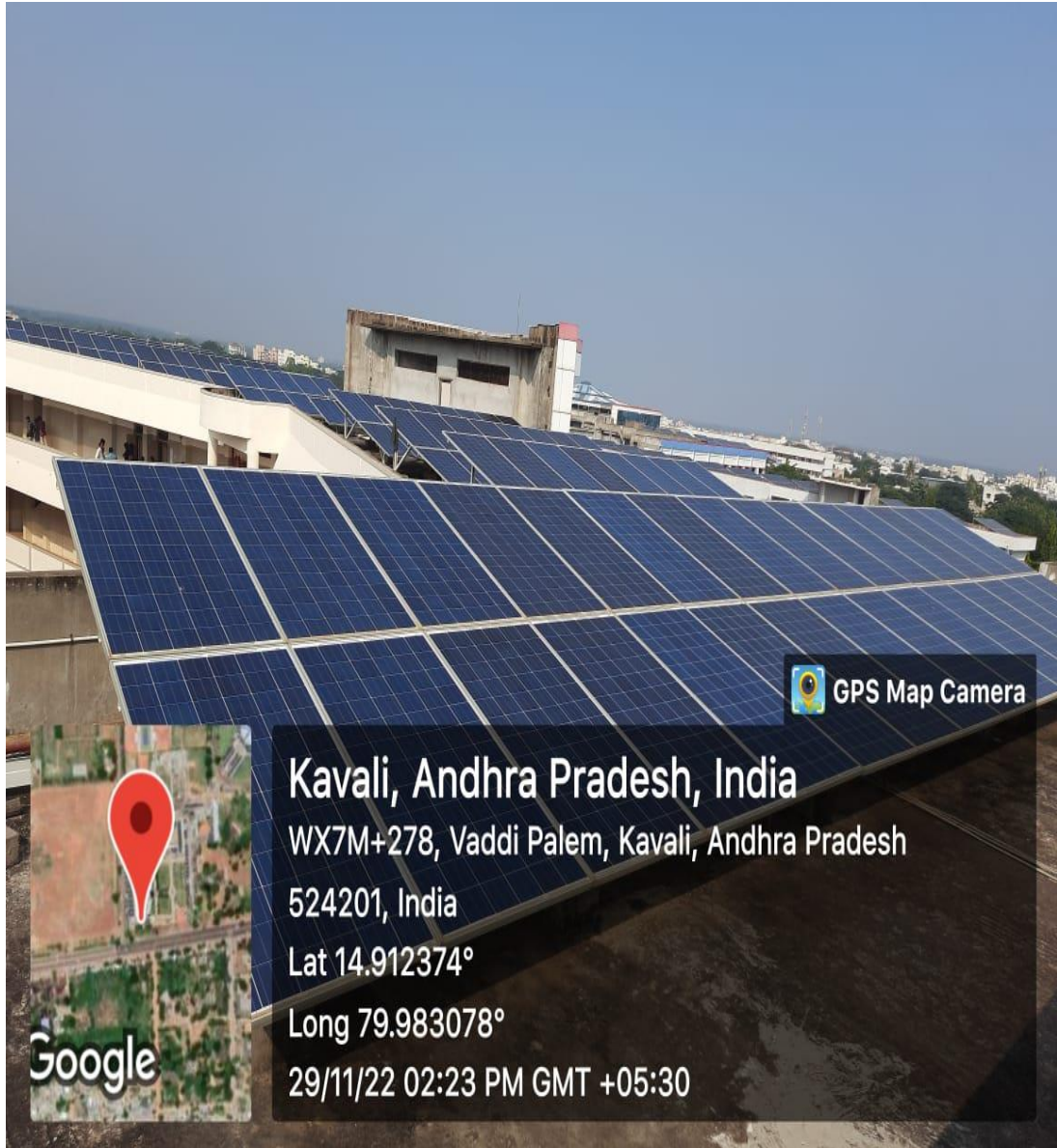
Figure: Grid Connected Solar Plant
