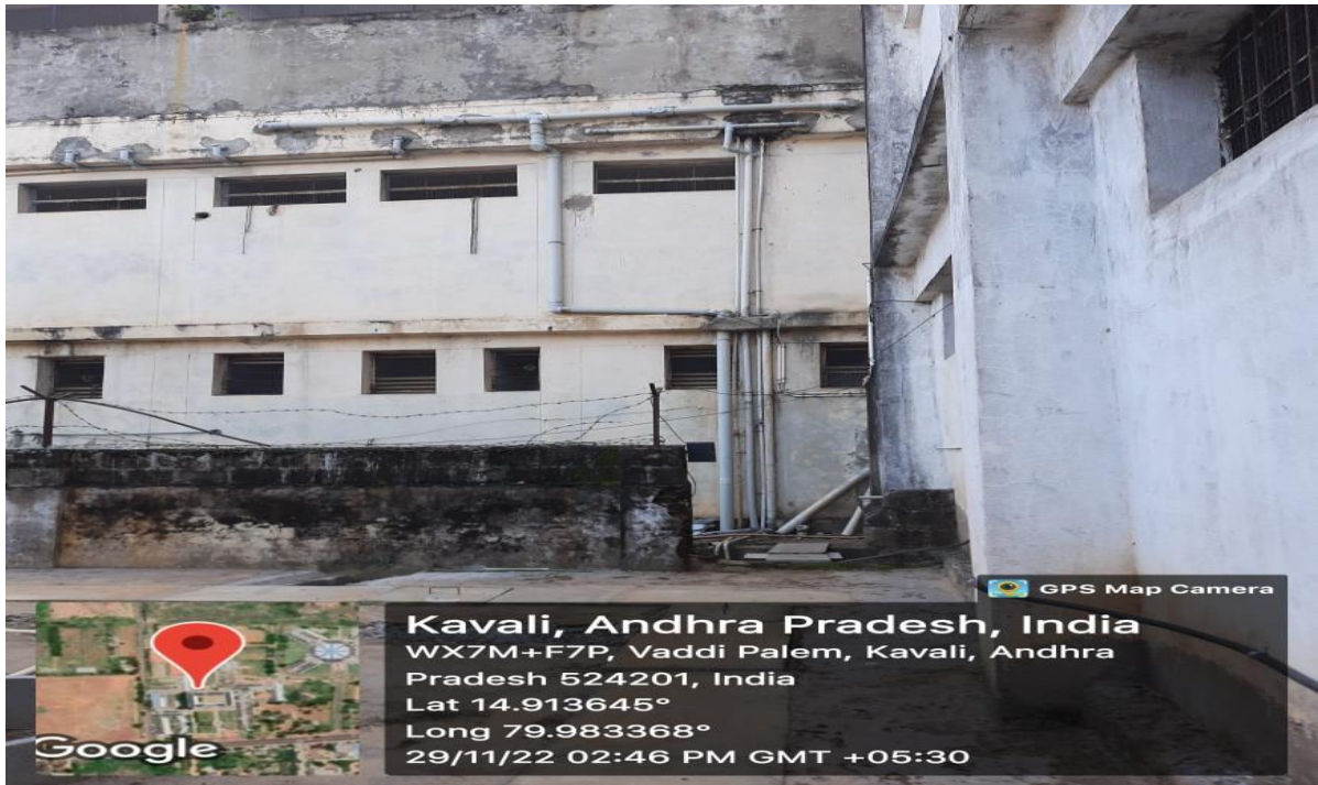
Figure: Rain Water Storage External Pipes
