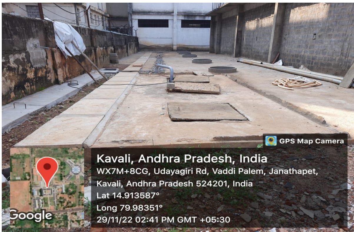
Figure: Rain Water Harvesting
